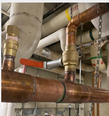
Approximately 160 domestic water valves and 80 heating valves have been abated and replaced
