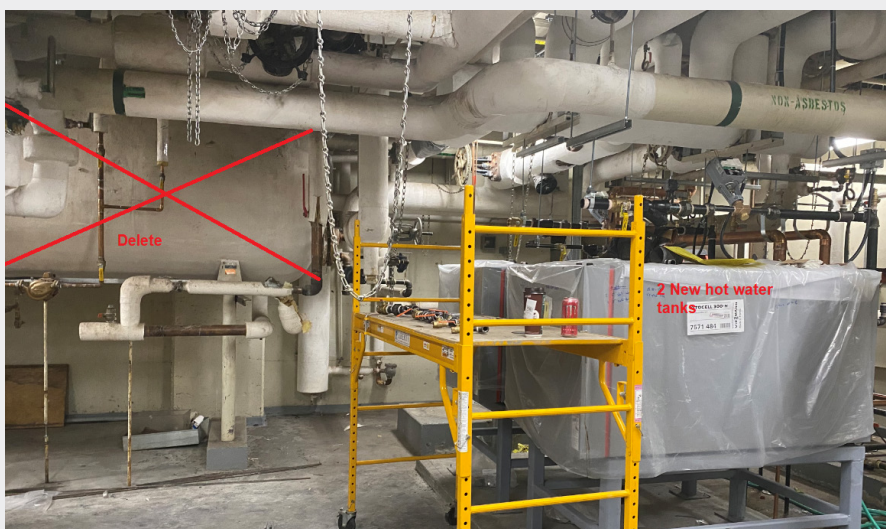
Existing hot water tank to be removed and new tanks ready for installation
