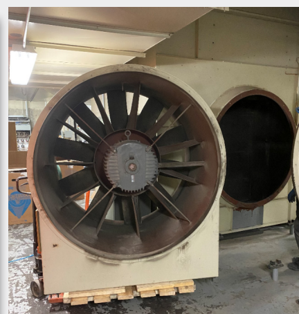
One of four rebuilt main building ventilation fans
